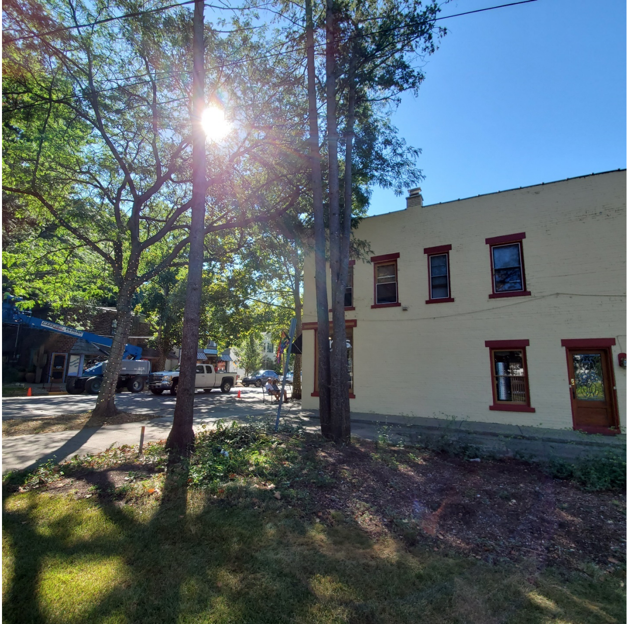
Figure 2: Mulch bed and tree removal along southern side of Village Square Park
