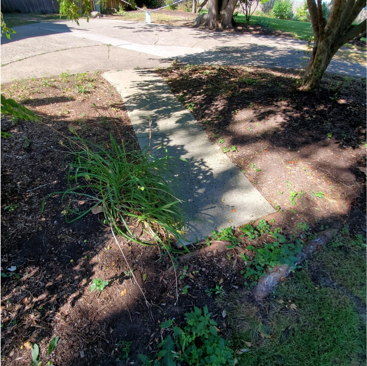
Figure 6: Needed concrete removal of walkway in southwest corner
