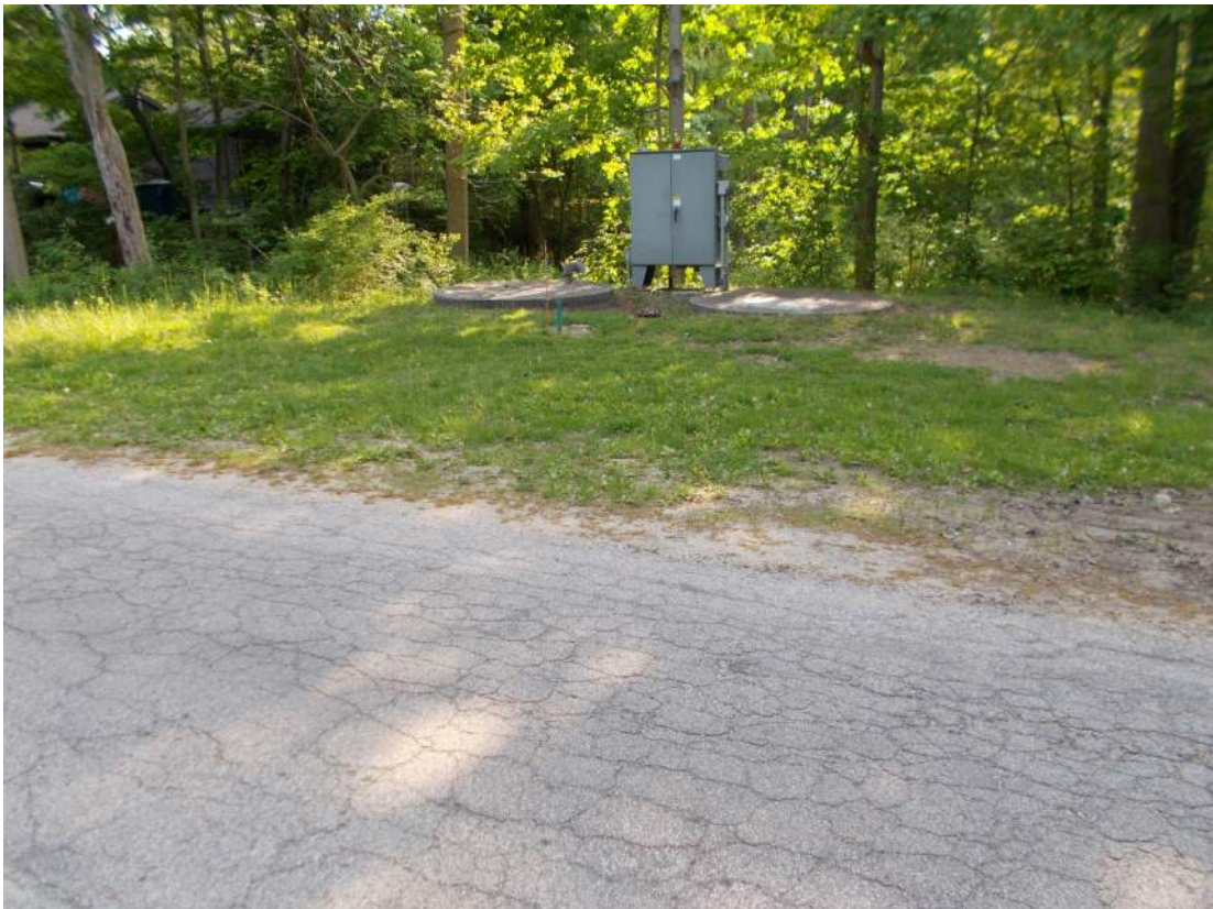
Wastewater lift station on west side of Maple Street north of Mason Street
