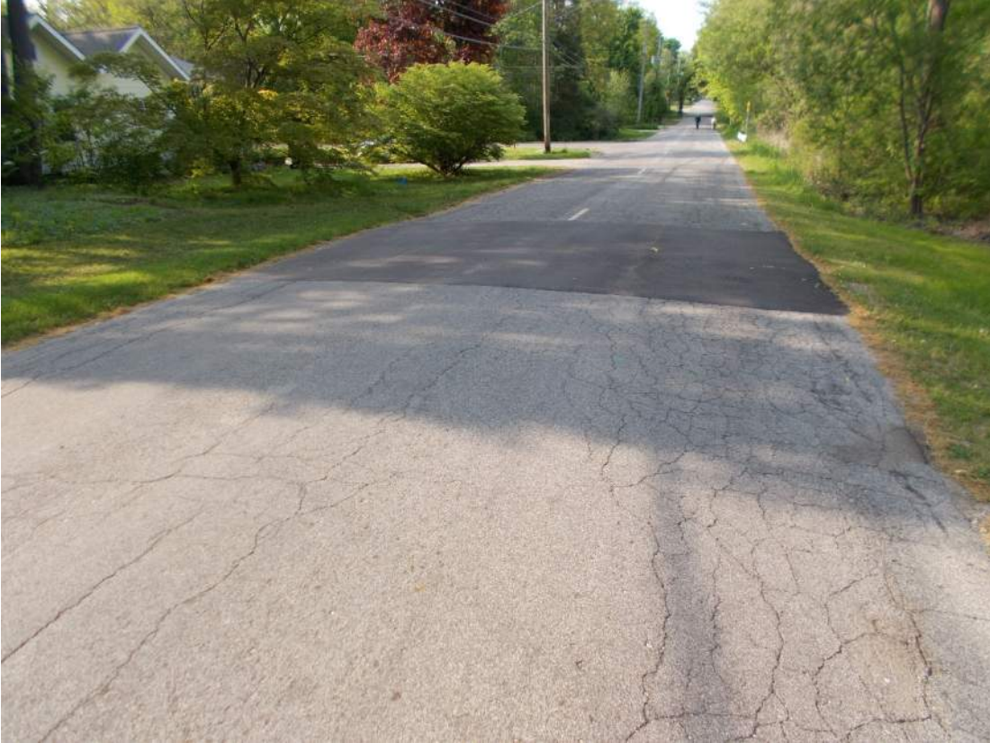
Patch from 2022 water main break on Maple Street south of Mason Street
