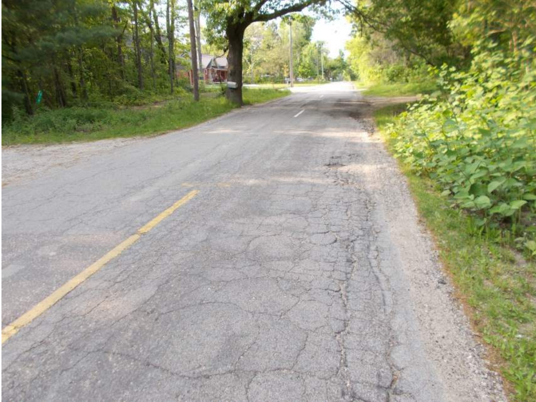
Failed pavement on Maple Street north of Mason Street looking north
