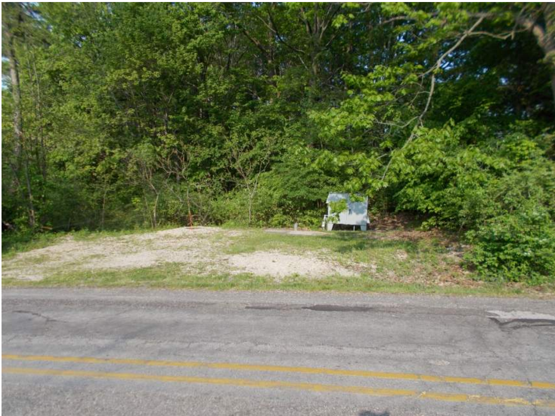
Wastewater lift station on east side of Maple Street south of North Street
