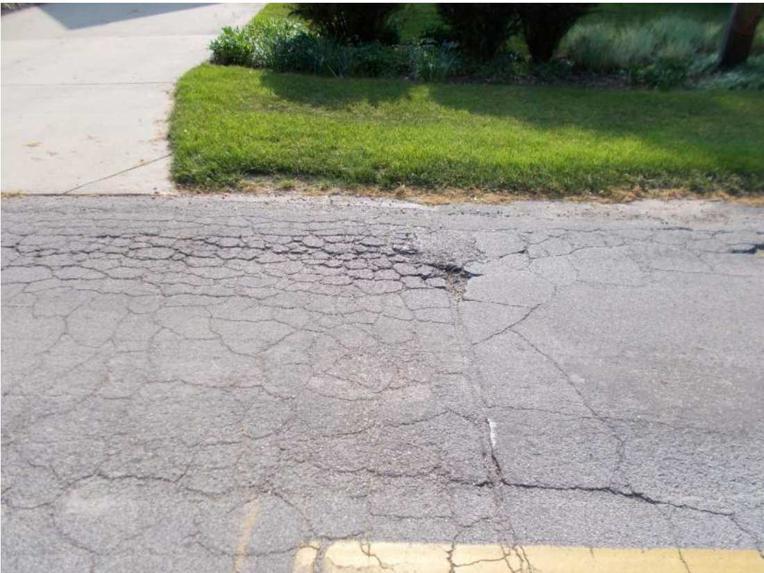
Failed pavement on Maple Street north of Allegan Street looking west
