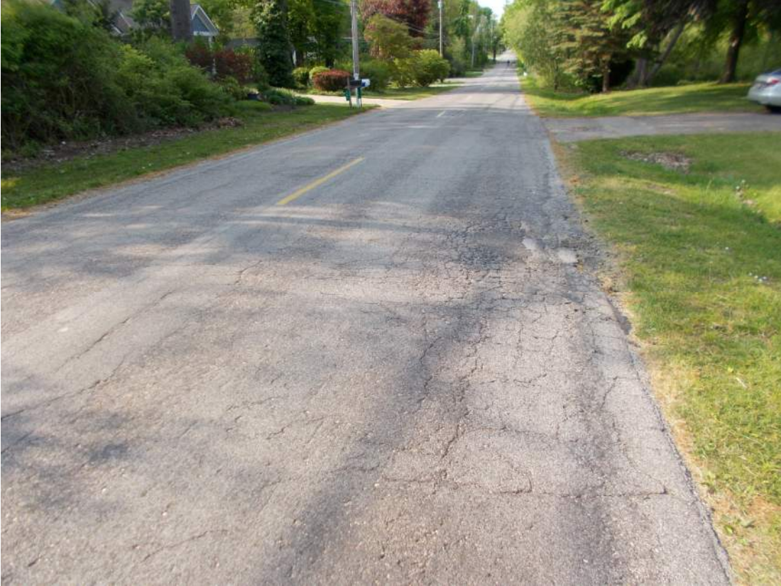
Failed pavement on Maple Street north of Allegan Street looking north
