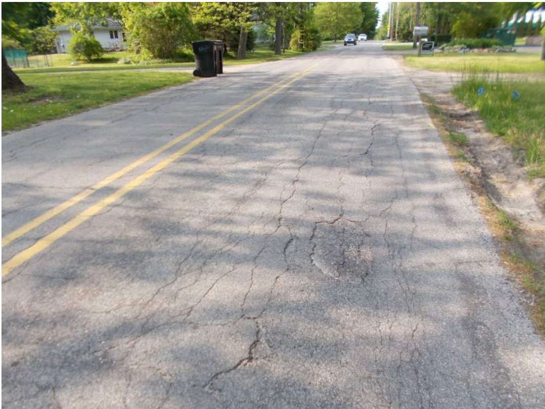
Failed pavement on Maple Street north of Blue Star Highway
