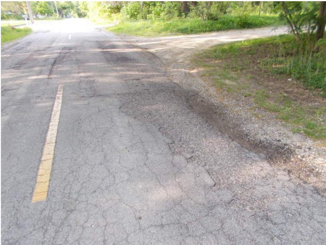
Failed pavement and slurry seal on Maple Street north of Mason Street looking north
